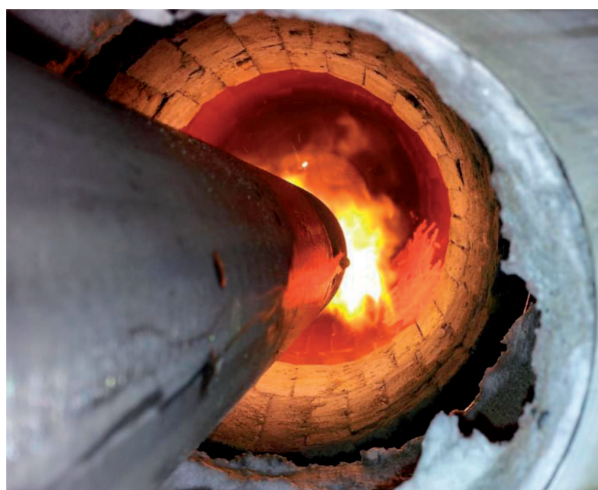
Fig. 2. Rotary kiln equipped with oxygen burner
